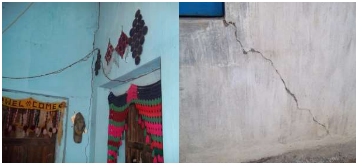
Picture 5.11: Blasting Effect on Housing Pattern at Langijoda village near lingaraj open mines
